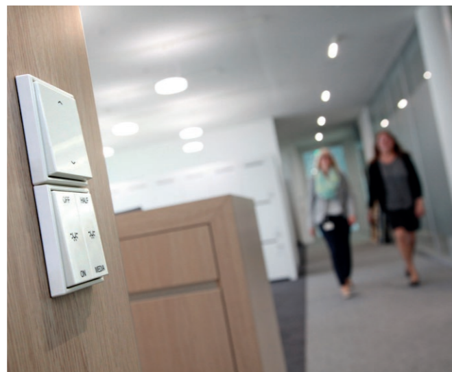
Over 500 of the company's own pushbutton modules ensure optimal working conditions in the ZF Forum.
